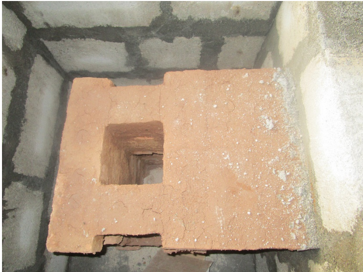
Figure 8: Combustion chamber of the Ahotor oven
