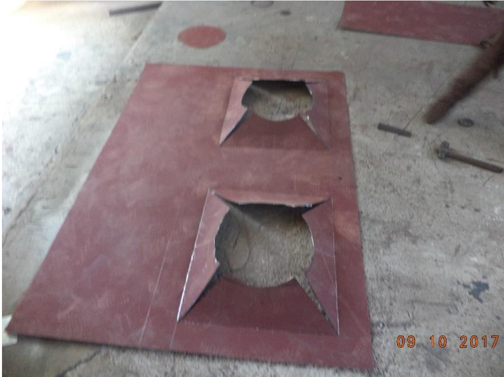
Figure 15: Molding of Fan duct threshold
