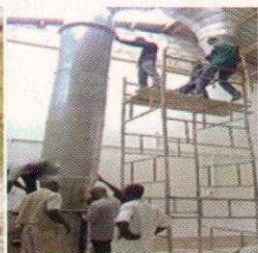
Coupling Cyclone to Blower
